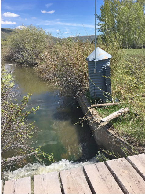
Site 1, 10' parshall flume and stilling well
