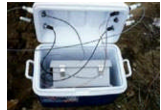
Enclosure is sealed inside of a plastic cooler, to protect it from vandalism.
